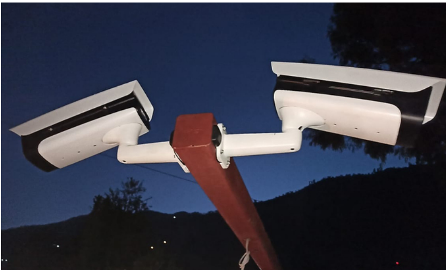
The CCTV cameras installed by the police in Kullu. Tribune Photo
